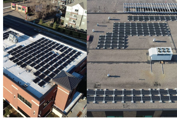
Explore Connected Campus-Wide Renewable Infrastructure
