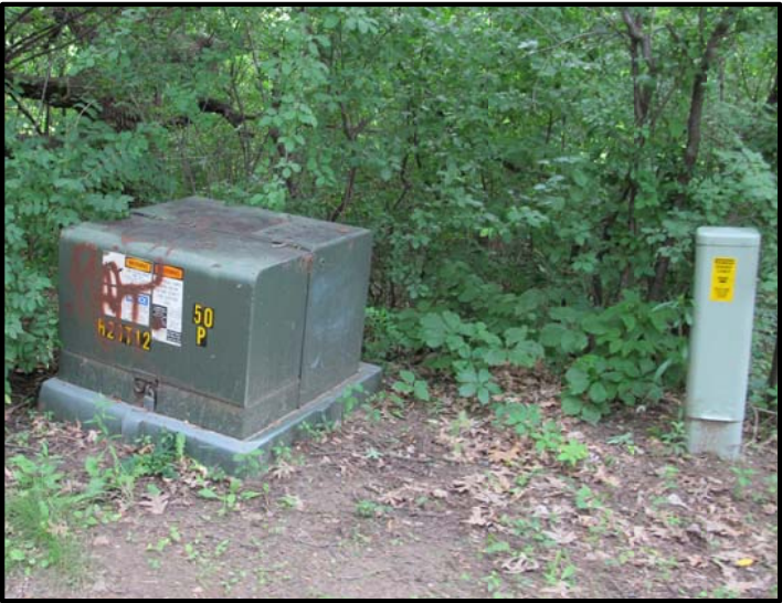
2 EXISTING TRANSFORMER PHOTO SCALE: NONE
