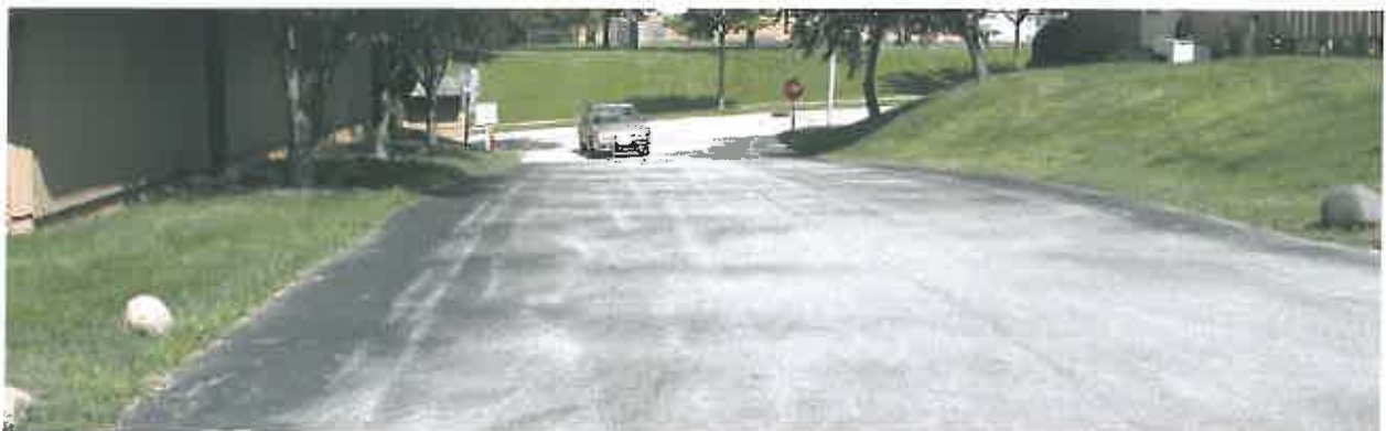
Gray asphalt pavement shows through where sealcoat has worn off the driveway of an apartment complex.
